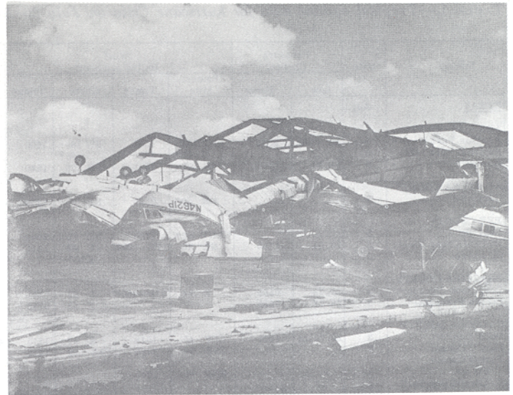
FIGURE 4.—Hurricane Celia damage at the Corpus Christi International Airport (Official National Ocean Survey Photograph).
