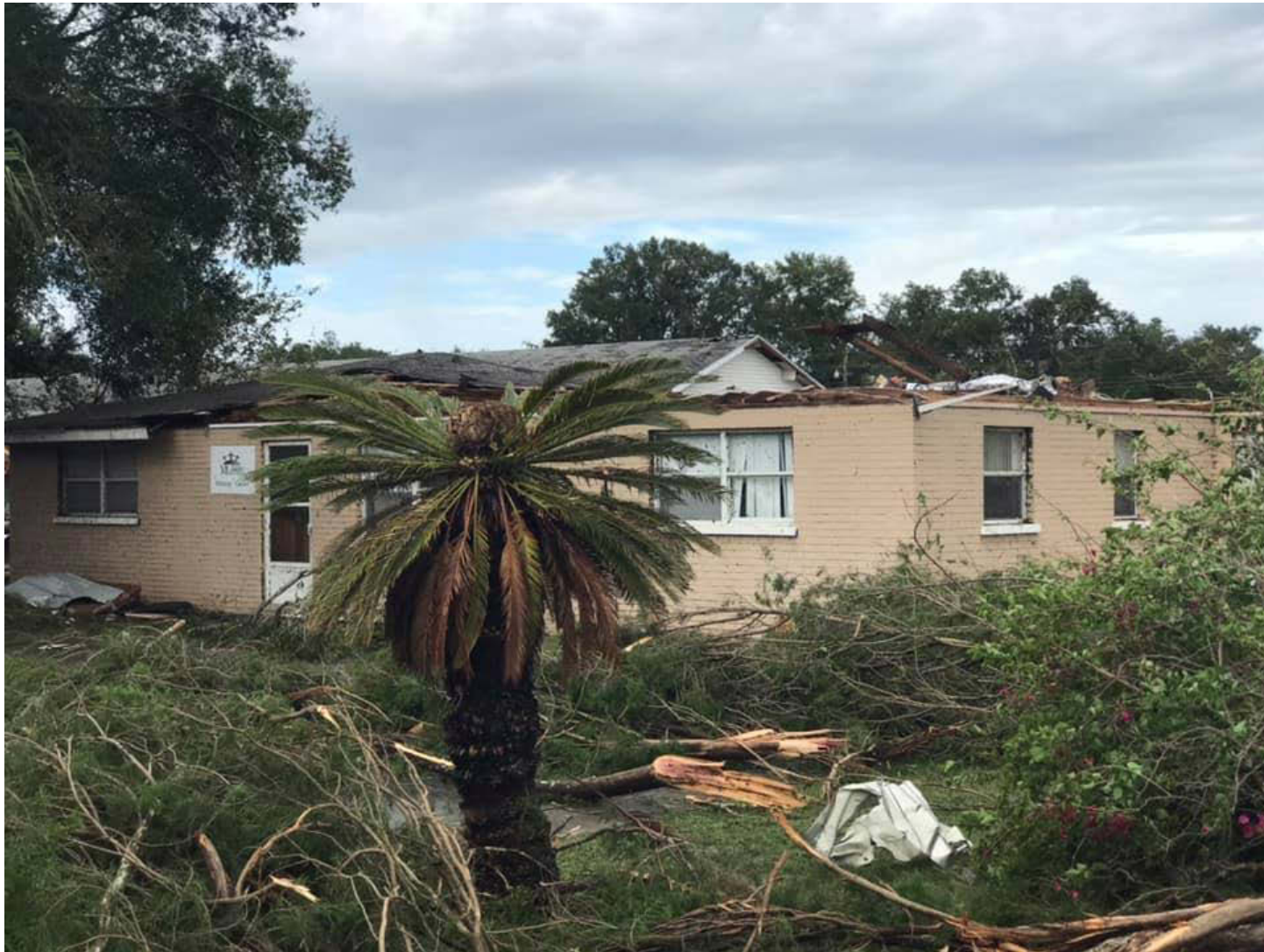
Figure 4. Tornado damage to a home in western Polk County, Florida (Courtesy NWS WFO Tampa Bay).
