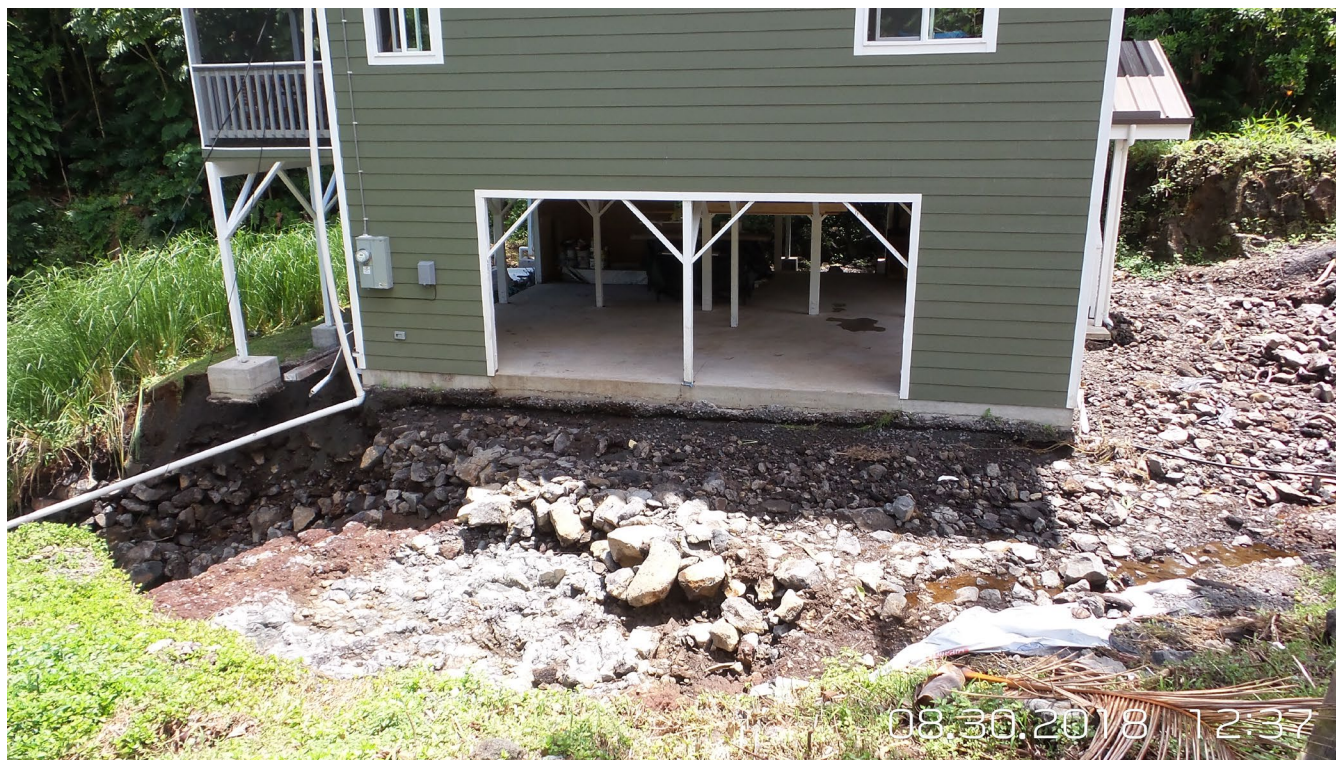
Figure 5. Flood damage to a property in Hilo on the Island of Hawaii.
